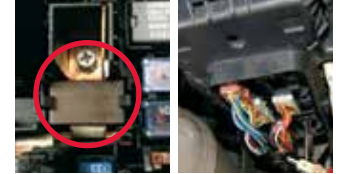
Figure 12 ELD bottom fuse box
